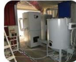
Feeding system and heat exchanger
